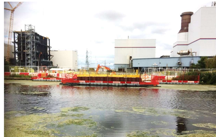
Figure NTS12: Typical cofferdam that would be required on the canal, adjacent to the intake for Keadby 2 Power Station
